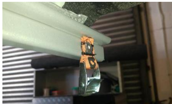
Figure 12: Buckle strap riveted onto awning arm
